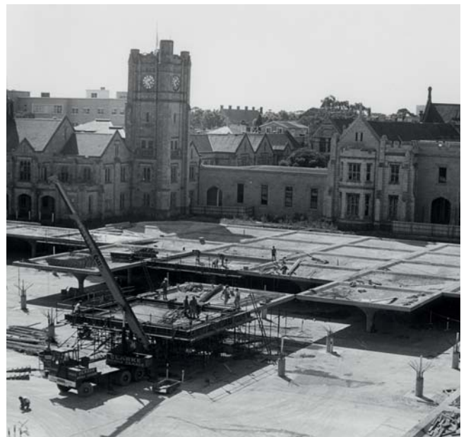
Carrick Chambers, Construction of the car park under the south lawn, taken from the east tower of the John Medley building, 1972. Property and Campus Services Photographic Collection, University of Melbourne.
